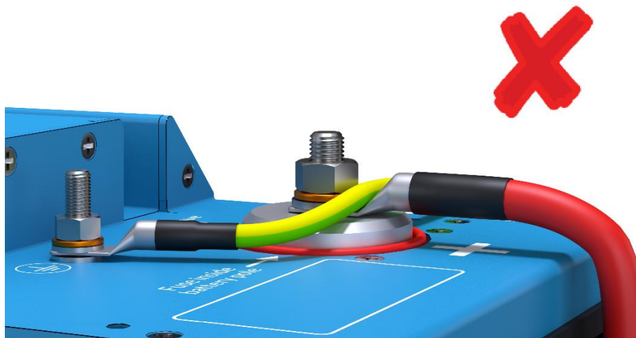
Figure 17 - Wrong routing of equipotential bonding wire
